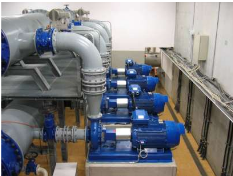
Figure 3 Installation of several pump-turbines in parallel when high flow rate fluctuations are expected.
